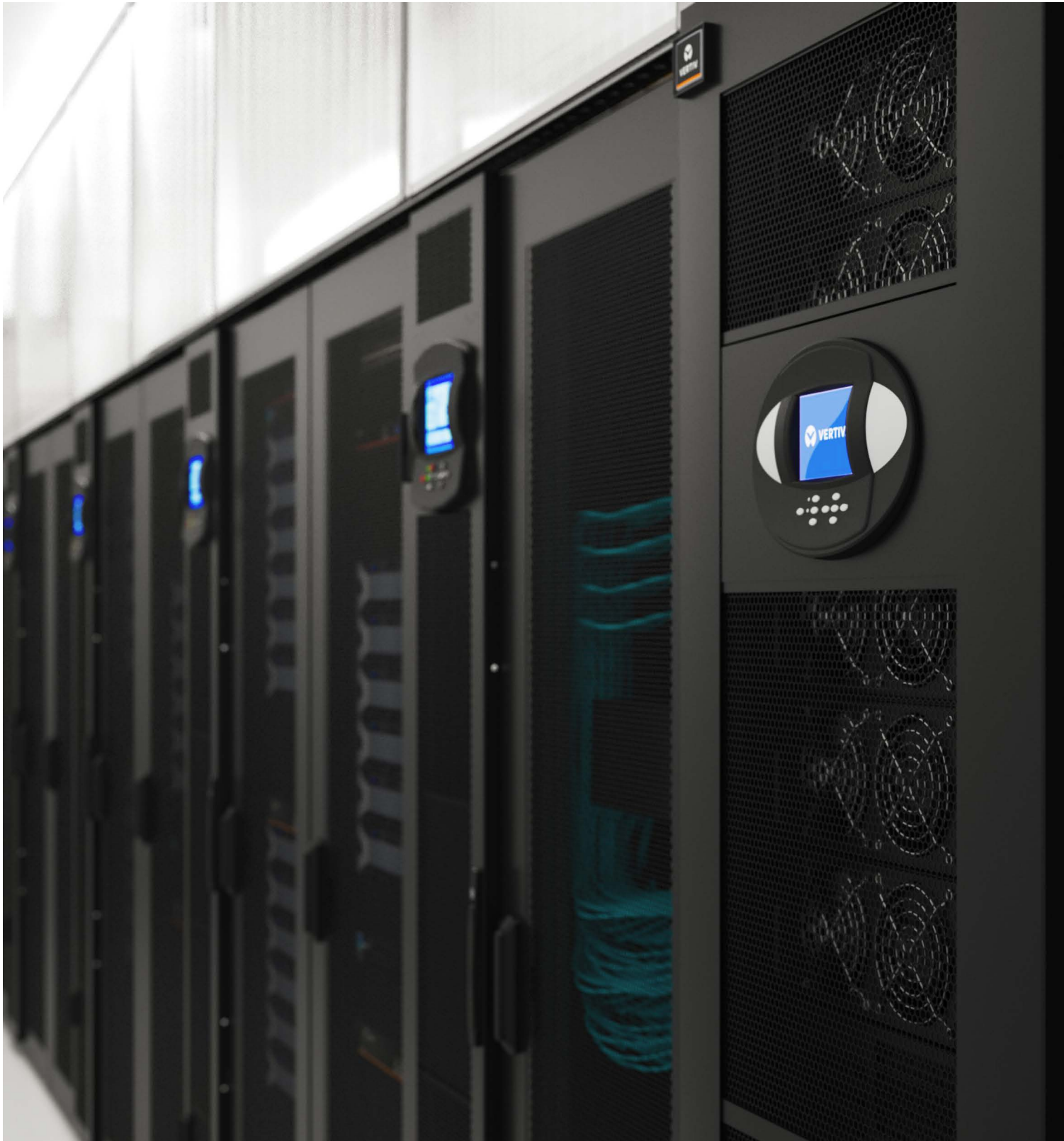
Interior view of Vertiv™ SmartMod™
